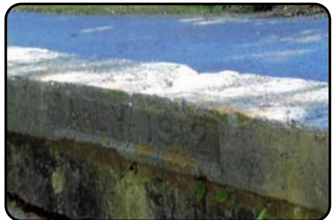
About 1/2 miles from the parking lot on E. Main Street there is still a cement bridge built by Logan Valley now used as private driveway. PHOTO 6
